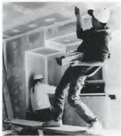
Julian Wong '95 shows great style as he spackles the ceiling of a Habitat house while Mariah Howe '94 works on the walls.
